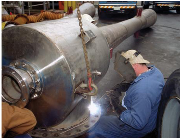
A welder modifies newly designed jets that spray steam into the condensers at The Geysers geothermal power plant. With a 750-megawatt output from 14 units, The Geysers is the largest producer of geothermal power in the world.
